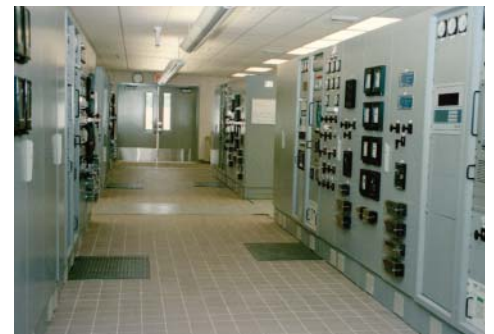
Gas Turbine Controls
