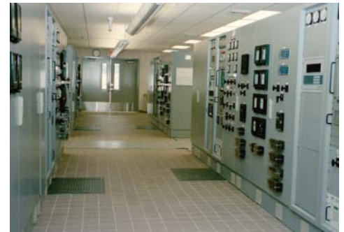
Gas Turbine Controls
