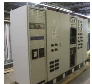
Gas Turbine Control Panel
